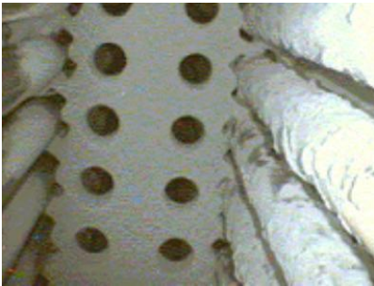
Fig. 2 Photo of tube fouling (hot leg on the right side) – Source EDF CEIDRE
